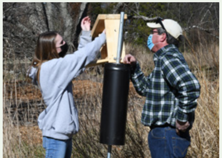
Girl Scout Sydney Sheffield is assisted by her father with the installation of ten bluebird houses she built for the Garden.
